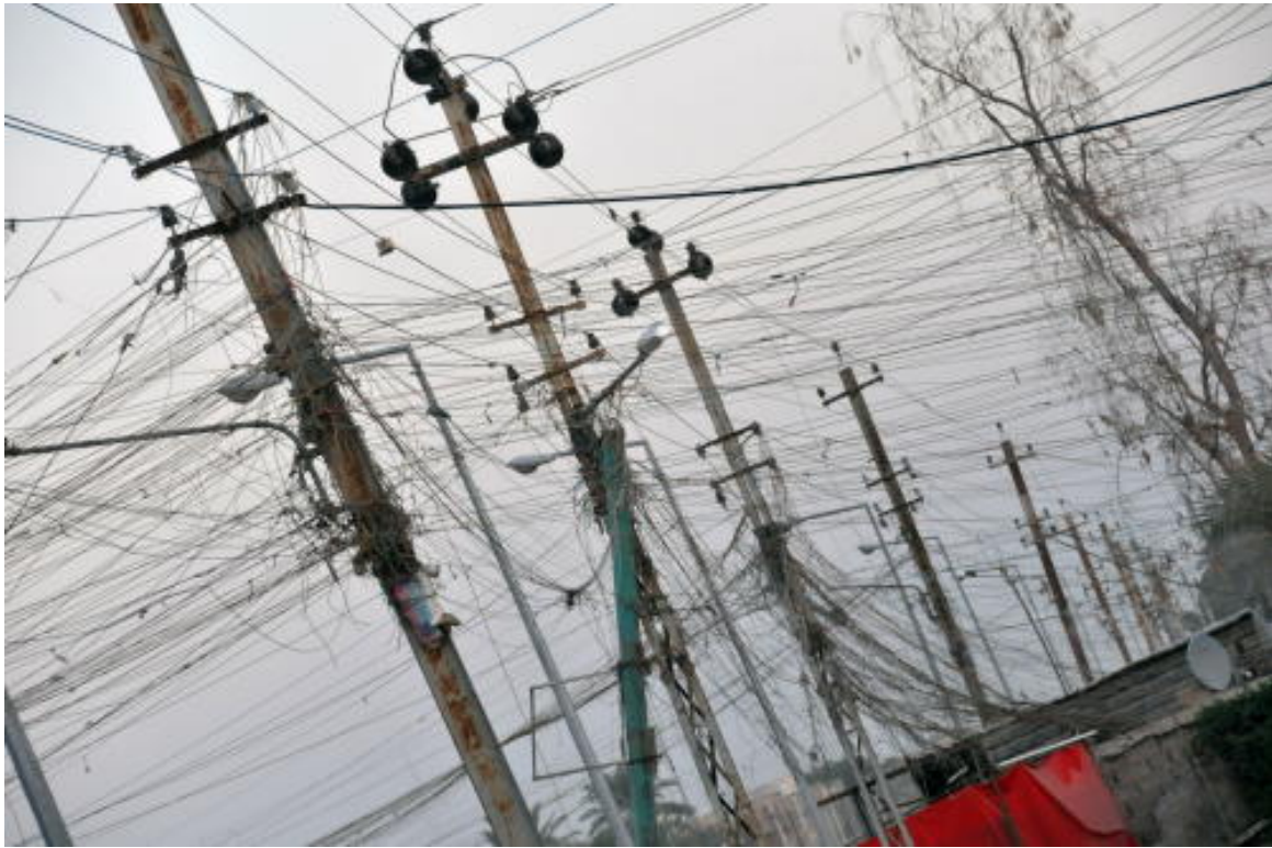
Figure 12. Electrical Wires in Adhamiyah 179
